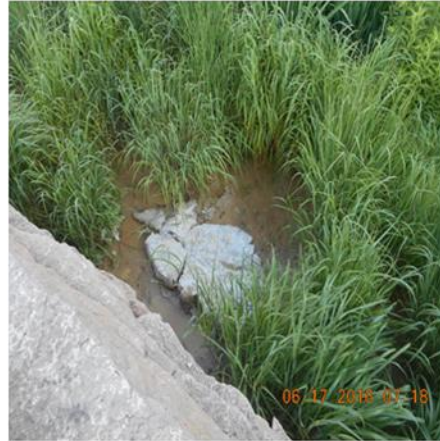
SEDIMENT BUILDUP IN AREA OF HDS OUTLET PIPE
