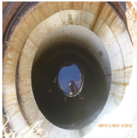
VIEW OF TURBID WATER IN HDS
