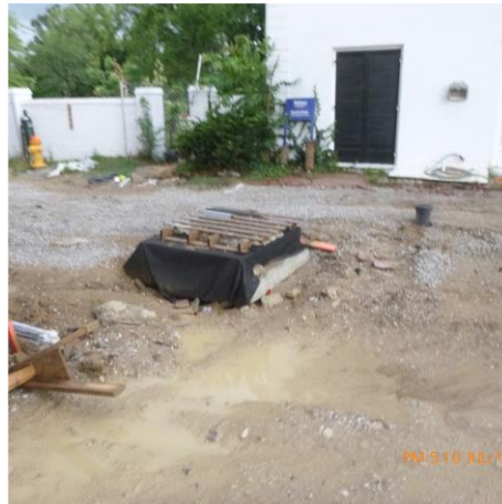
INLET PROTECTION NPLACE
