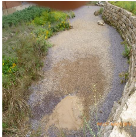
SEDIMENT ENCROACHMENT INTO RAIN GARDEN A
