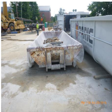
DUMPSTER FOR TRUCK WASH OUT
