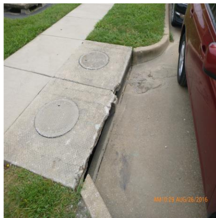
REPLACE MISSING INLET PROTECTION (GARDEN AVENUE)
