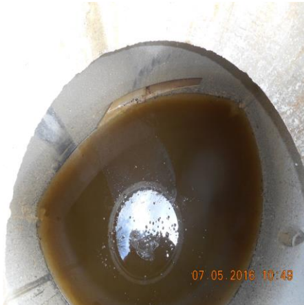
LOOKING AT TURBID WATER IN HDS
