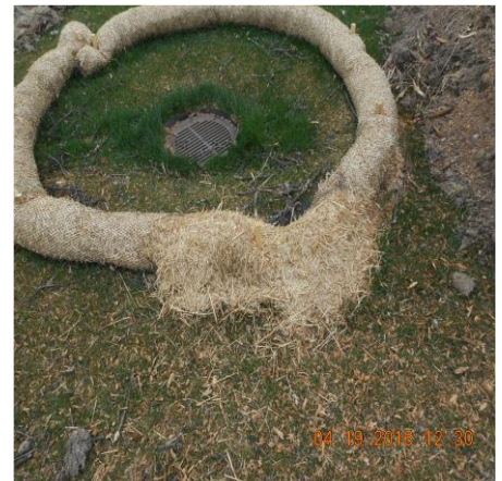
REPLACE TORN SILT SOCK AT GI 23K2-0444D
