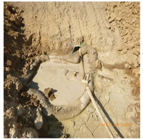
TURBID WATER BEING PUMPED DIRECTLY INTO STORM SEWER
