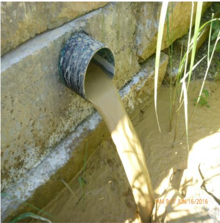
TURBID WATER FLOWING FROM HDS INTO BIODETENTION BASIN
