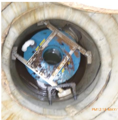
VIEW OF THE INSIDE OF DOWNSTREAM DEFENDER
