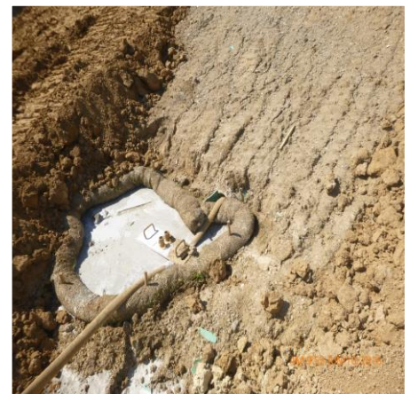
MONITOR SEDIMENT BUILDUP AT END OF PIPE
