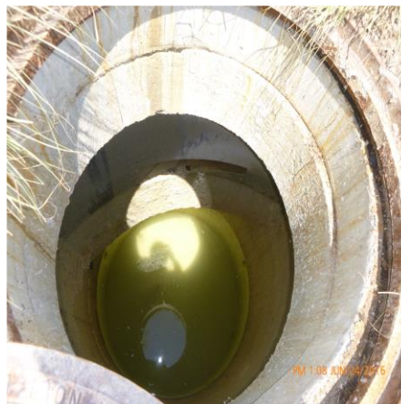
MONITOR SEDIMENT BUILDUP IN HDS – CURRENTLY AT 4"
