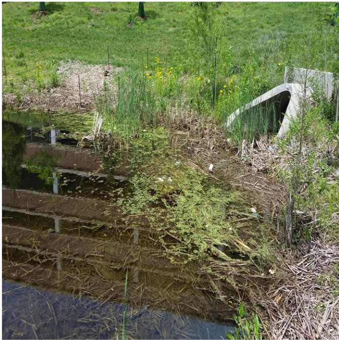
LOOKING NORTH AT INLET PIPE FES
