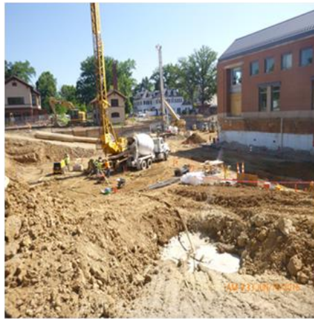
APPARENT SOURCE OF TURBID WATER AND SEDIMENT
