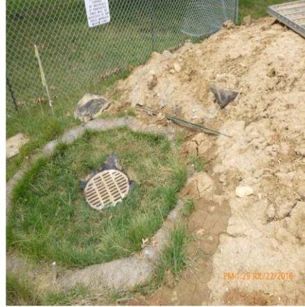
REPAIR OR ADD MORE SILT SOCK AROUND INLET
