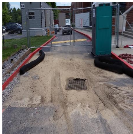
SEDIMENT ON PAVEMENT INDICATES PONDING AREA AT GI 23K2-0392D
