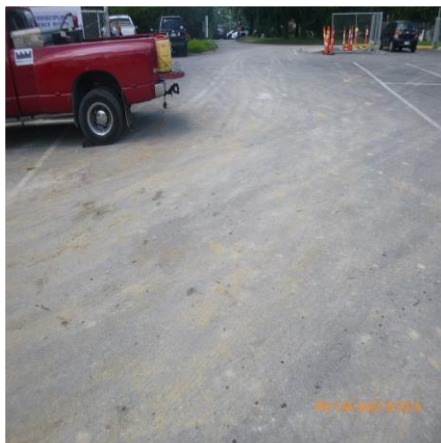
MONITOR SEDIMENT ON PARKING LOT LEAVING CONSTRUCTION SITE
