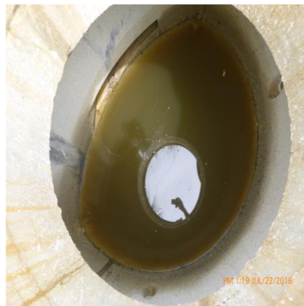
LOOKING AT TURBID WATER IN HDS
