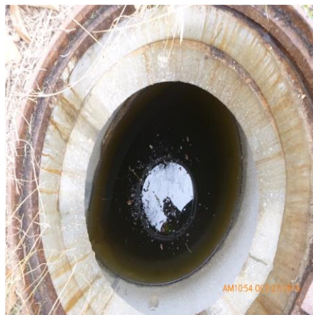
VIEW OF TURBID WATER IN HDS
