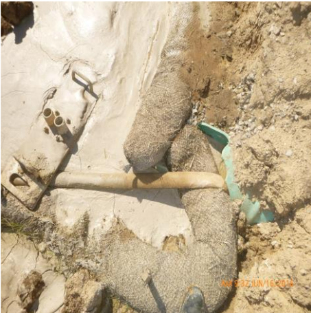
CLOSE-UP OF TURBID WATER BEING PUMPED INTO STORM SEWER
