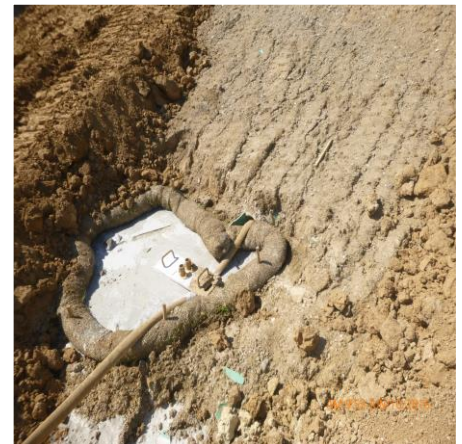
MONITOR SEDIMENT BUILDUP AT END OF PIPE
