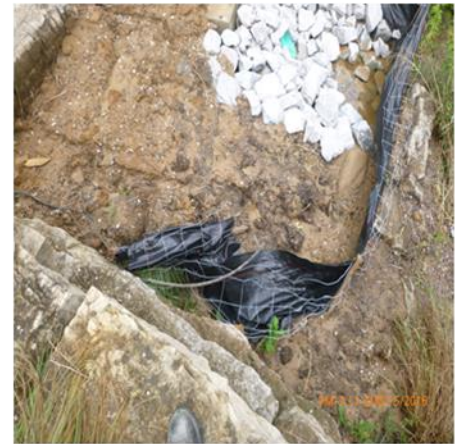
REPAIR UNDERMINED SILT FENCING BELOW DOWNSTREAM DEFENDER
