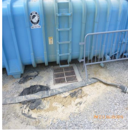
INLET # 1 & DEWATERING TANK
