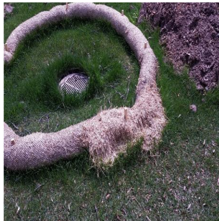
REPLACE TORN SILT SOCK AT GI 23K2-0444D
