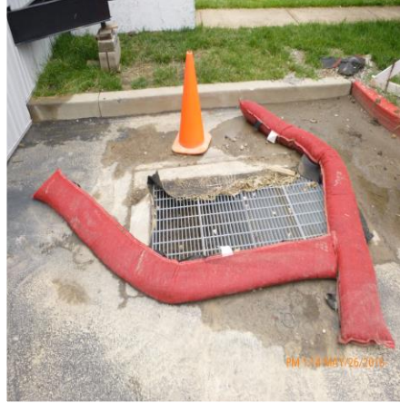
PIN OR WEIGH DOWN SILT SOCK AROUND INLET AT SE CORNER OF EAB
