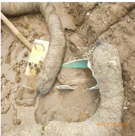
MONITOR SEDIMENT BUILDUP AT END OF PIPE
