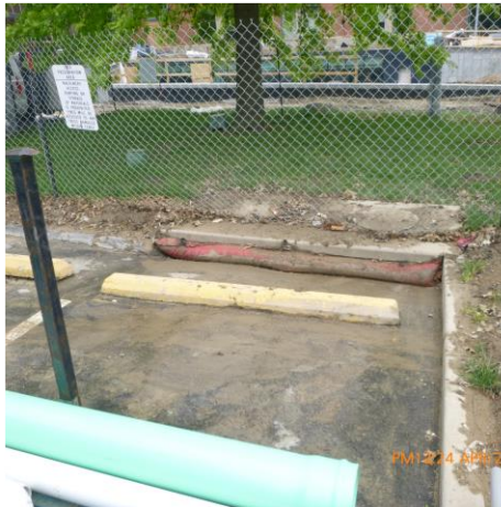
MONITOR SEDIMENT IN FRONT OF CURB INLET (PARKING LOT)
