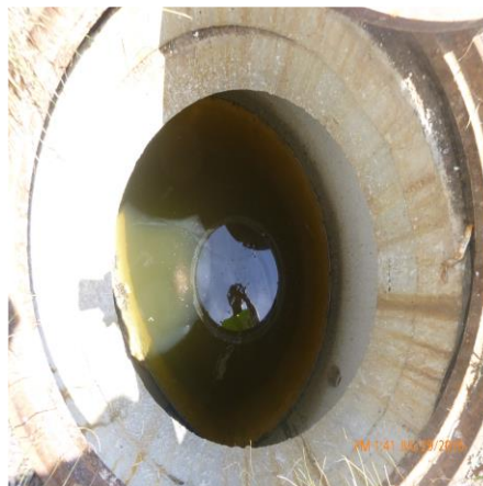
LOOKING AT TURBID WATER IN HDS
