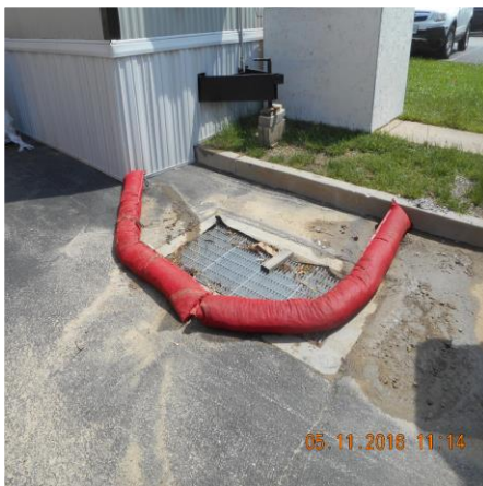
FILTER SOCK AT SE CORNER OF EAST ACADEMIC BUILDING
