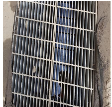
WATER STANDING IN GI 23K2-0392D INDICATES FILTER FABRIC IS CLOGGED
