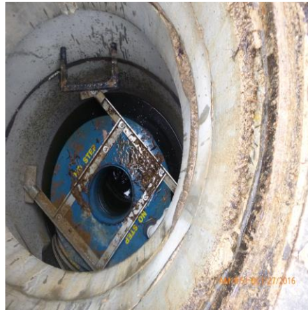
LOOKING AT TURBID WATER IN HDS
